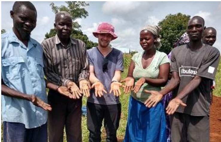
Many hands: Chris Markomanolakis, center, has raised over $3,000 for the Awach toilets and joined the big dig.
