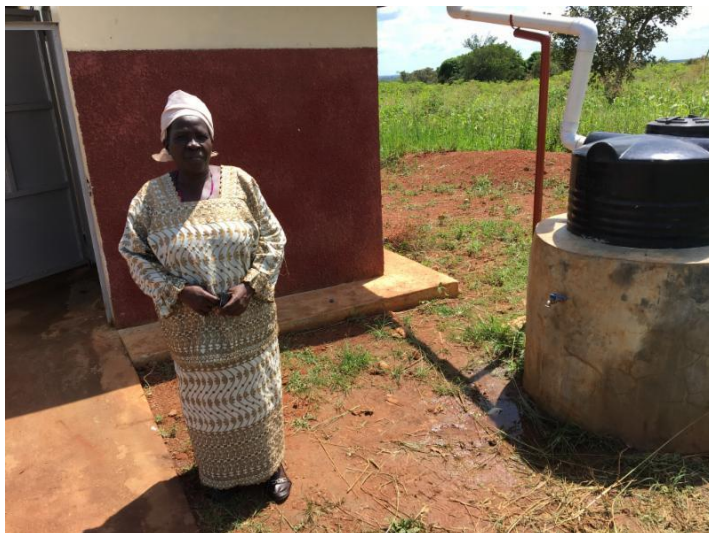
Christine Okot, Principal at the Ogul School, with her new toilets and hand-washing station.
